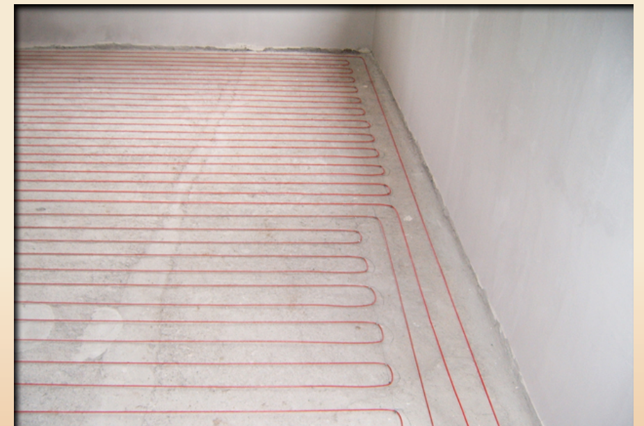
This shows two cables arranged on sections
